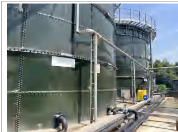
二级硝化/反硝化罐+一级硝化罐（接地罐体）
